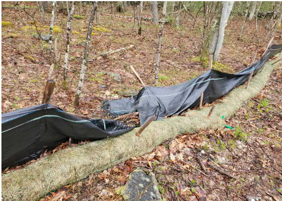
View of damaged silt fence in southern portion of the Site — facing south east
