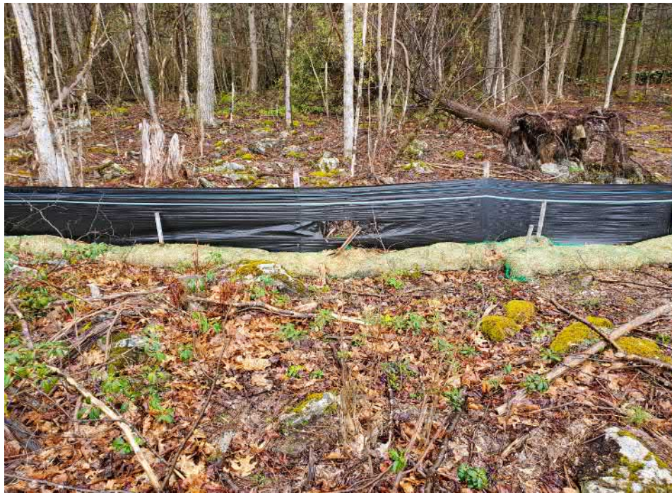
View of damaged silt wattle in north eastern portion of the Site — facing north
