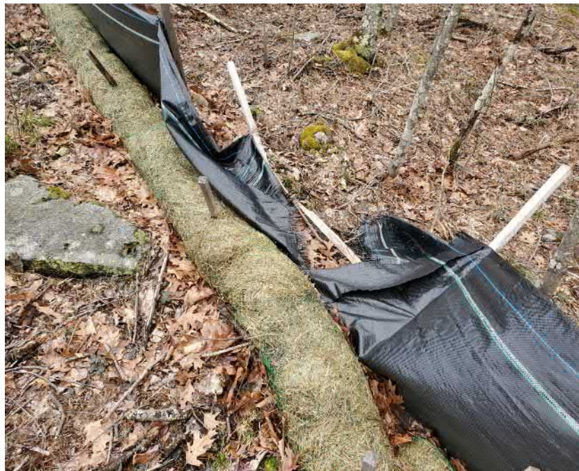
View of damaged silt fence in south east portion of the Site —facing north east
