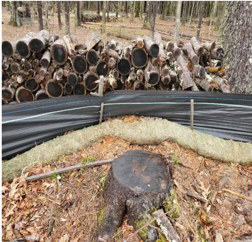
View of damaged silt wattle in northern portion of the Site —facing north
