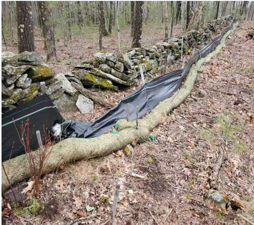
View of damaged silt fence in eastern portion of the Site —facing south east
