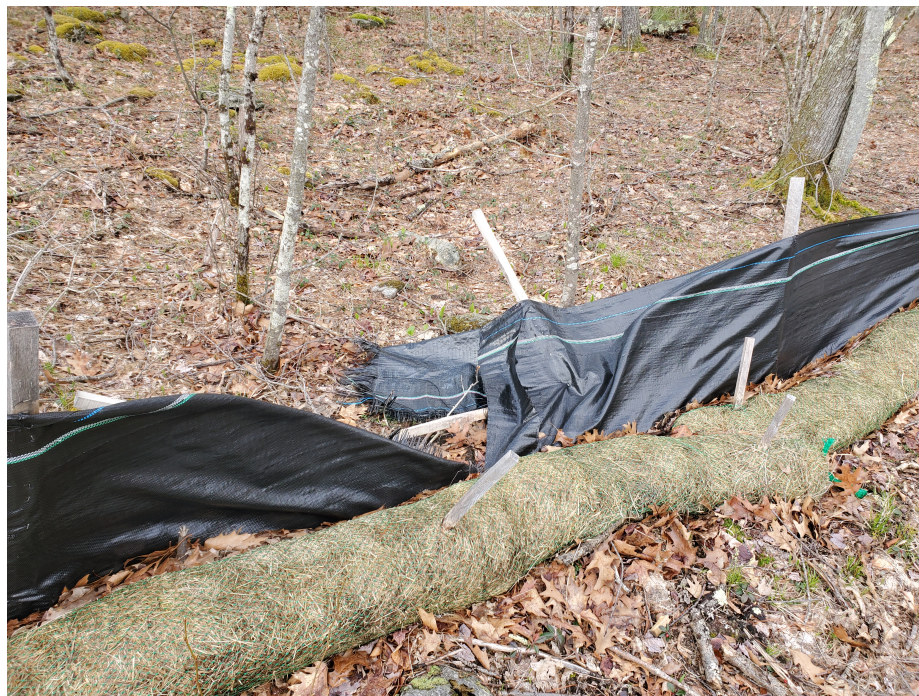
View of damaged silt fence in south east portion of the Site — facing south east
