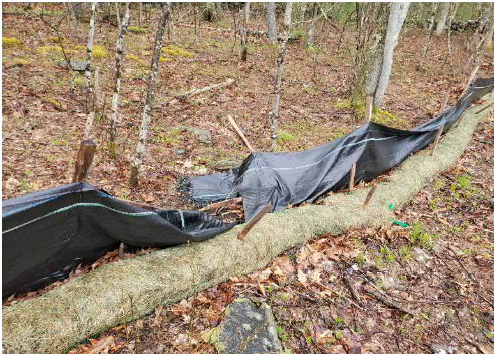
View of damaged silt fence in southern portion of the Site — facing south east
