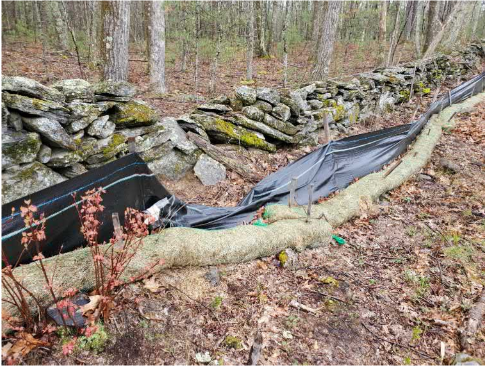
View of damaged silt fence in eastern portion of the Site — facing south
