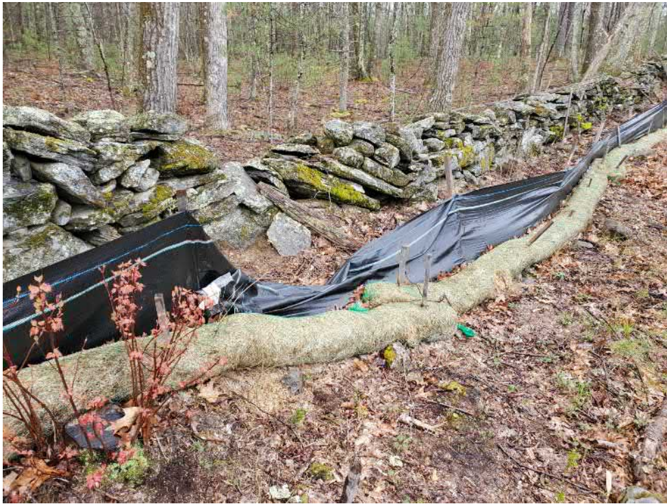
View of damaged silt fence in eastern portion of the Site — facing south
