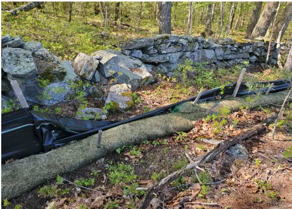
View of damaged silt fence in south portion of the Site — facing southeast
