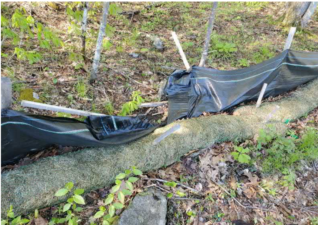
View of damaged silt fence in south east portion of the Site — facing south east
