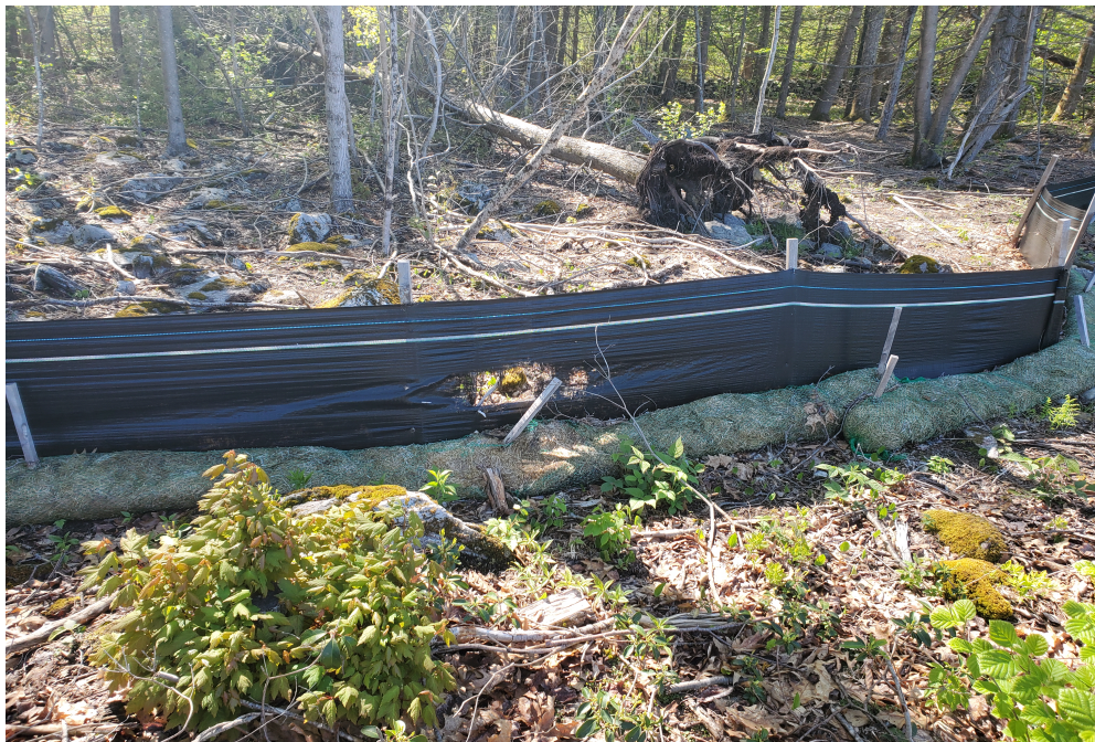
View of damaged silt wattle in north eastern portion of the Site — facing north east
