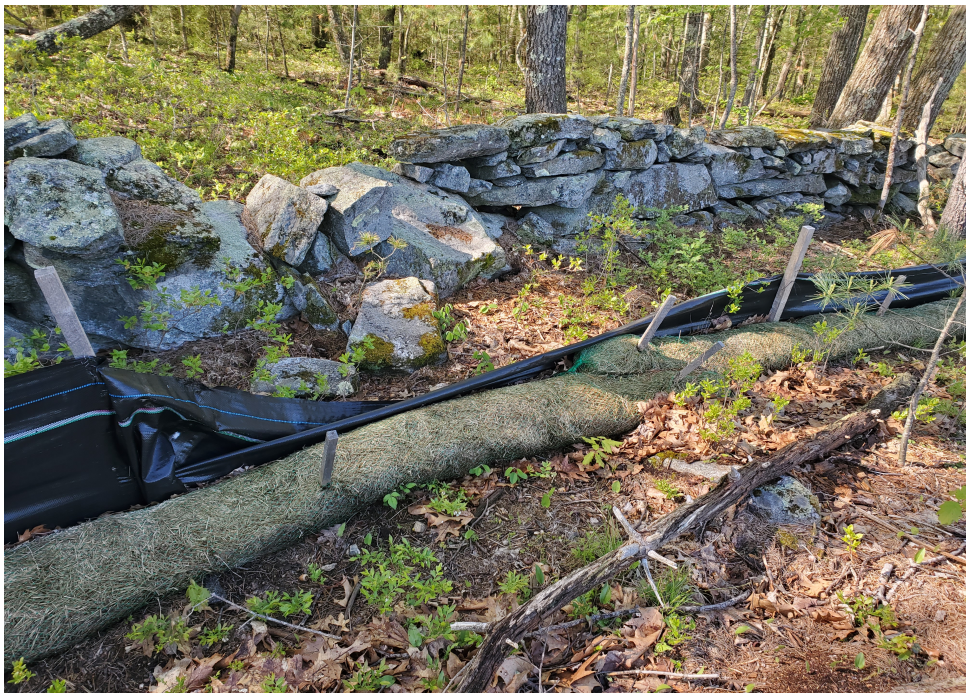
View of damaged silt fence in south east portion of the Site — facing south east
