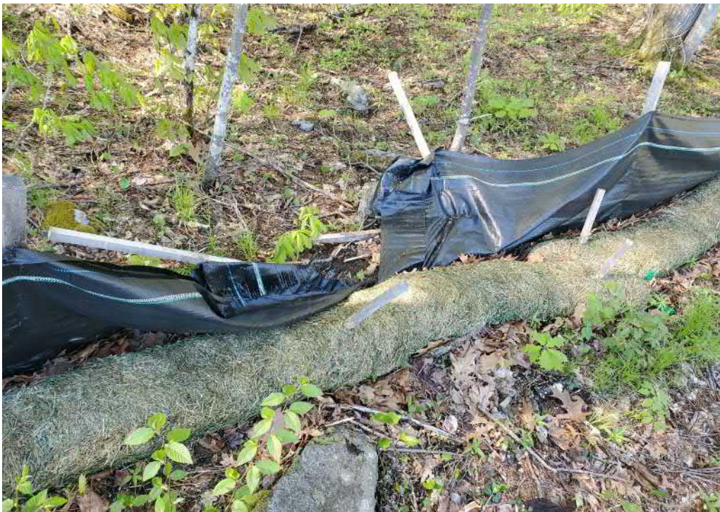
View of damaged silt fence in southern portion of the Site — facing south
