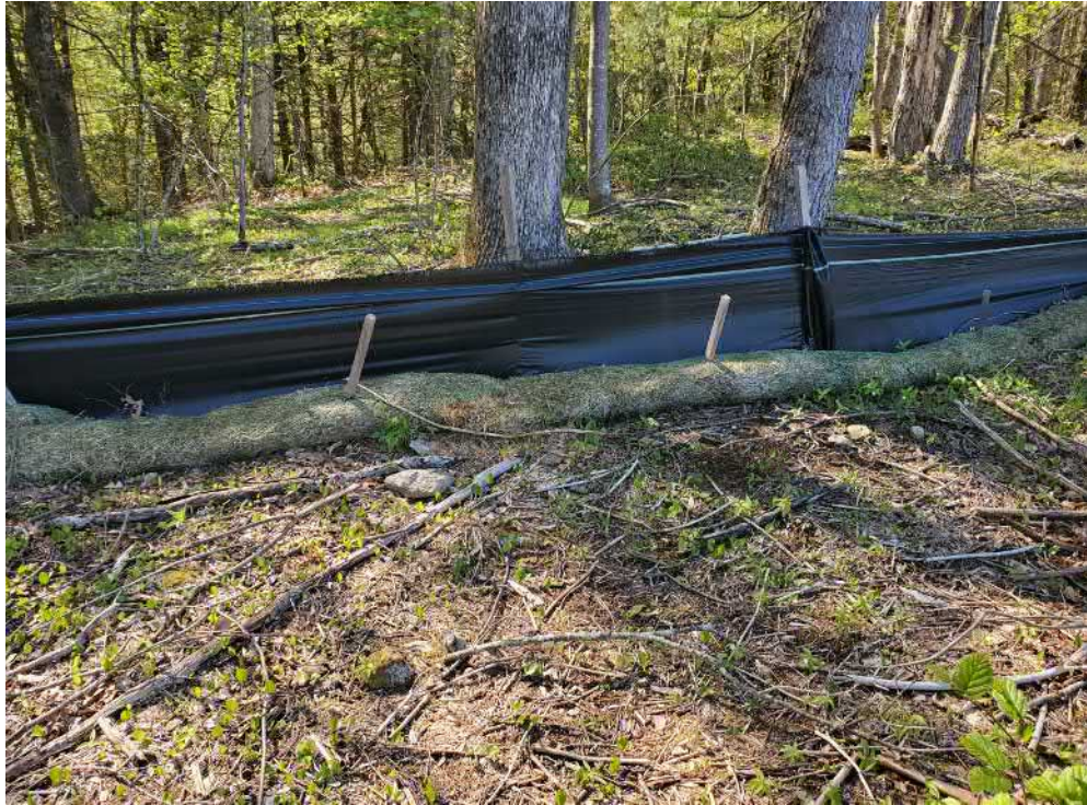
View of damaged silt wattle in northern portion of the Site — facing north
