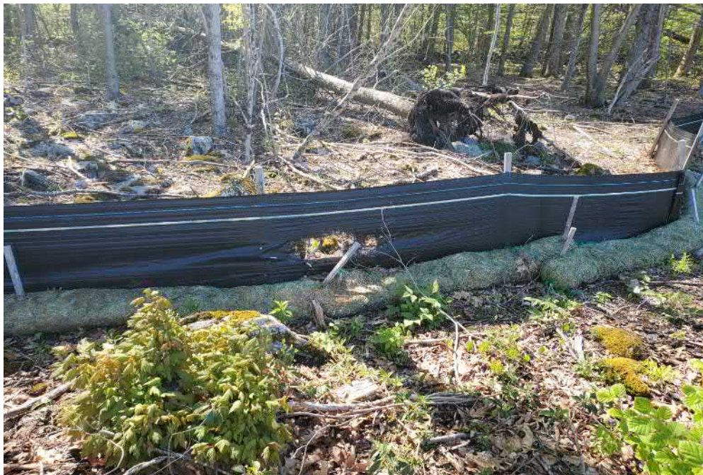
View of damaged silt wattle in northern portion of the Site — facing north
