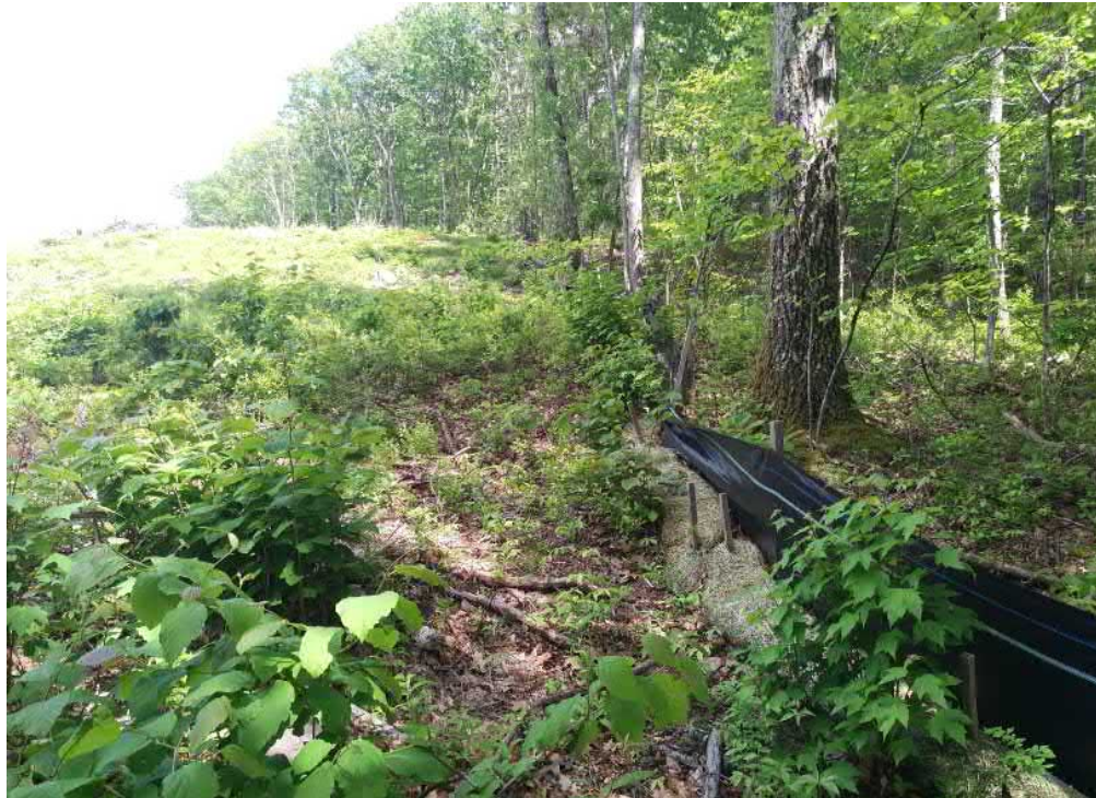
View of damaged silt fence southern portion of the Site — facing east
