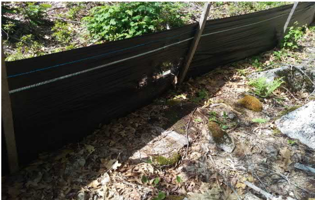
View of damaged silt fence northeastern portion of the Site — facing northwest
