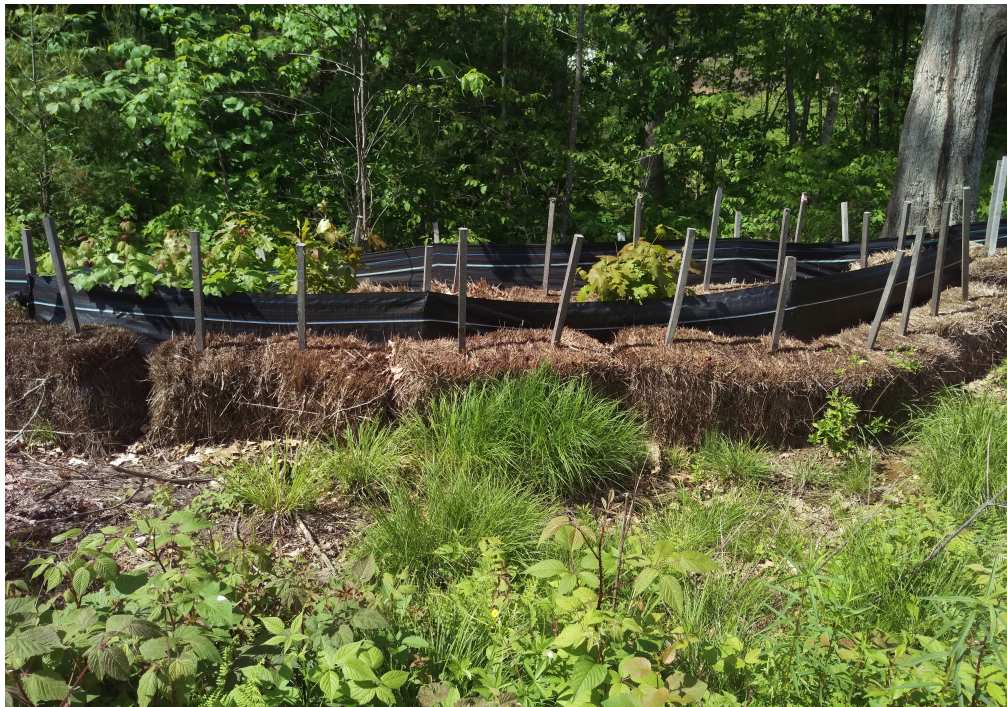
View of intact hay bales in northern portion of the Site — facing north
