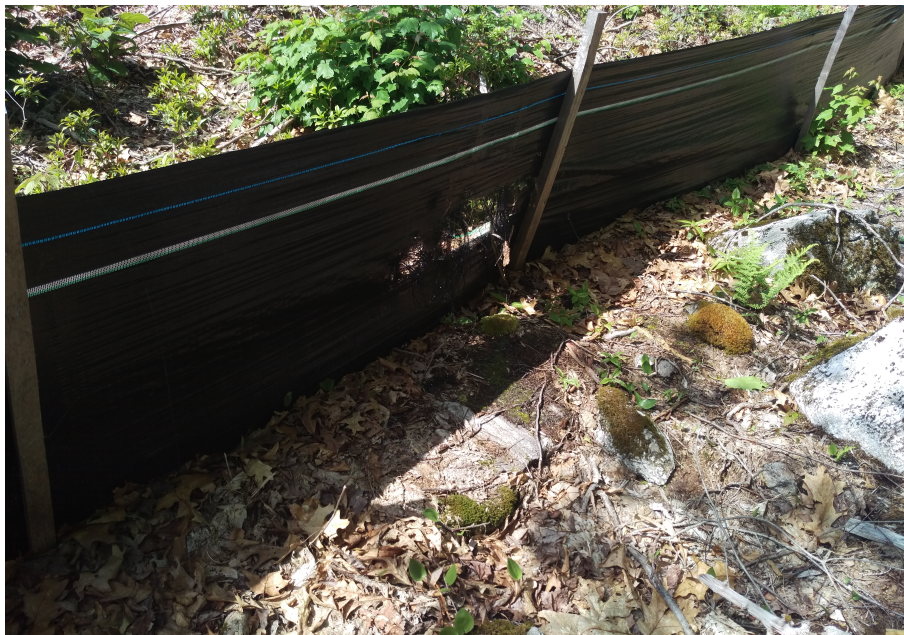
View of damaged silt fence north eastern portion of the Site — facing northwest
