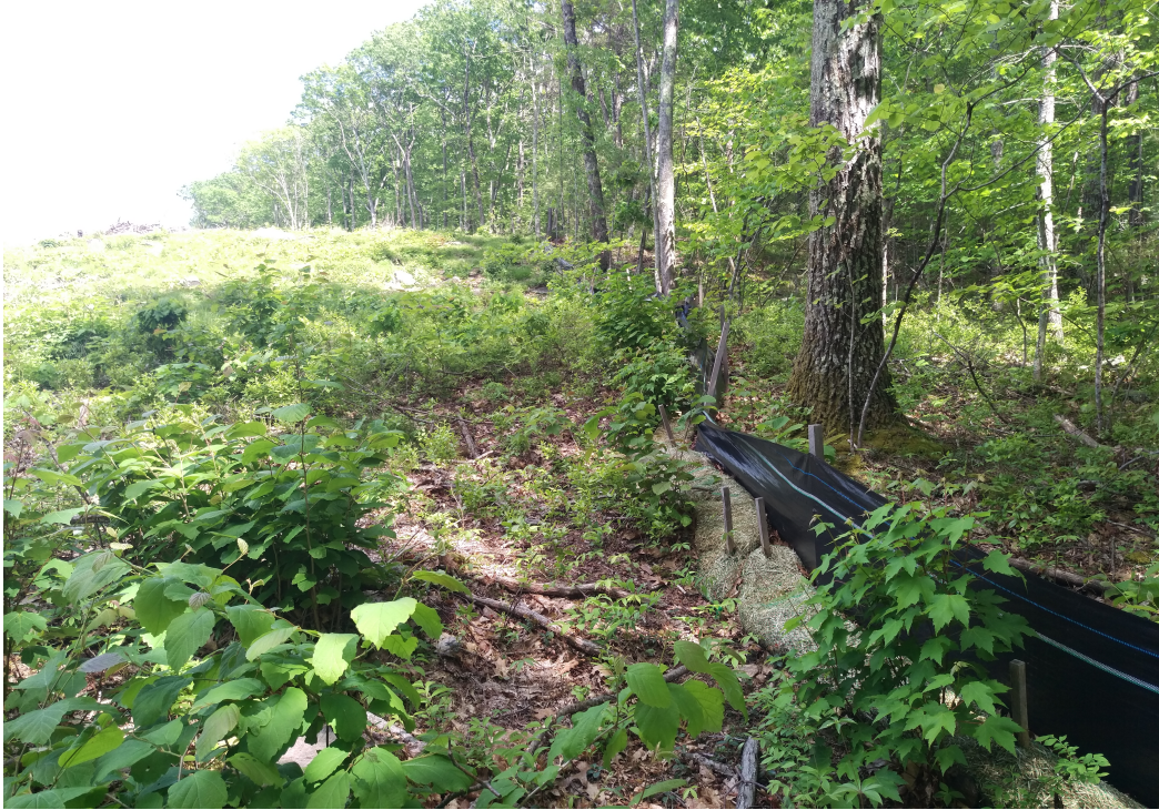
View of damaged silt fence southern portion of the Site — facing east
