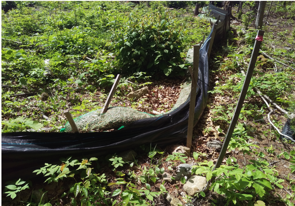
View of damaged silt fence in northern portion of the Site — facing north
