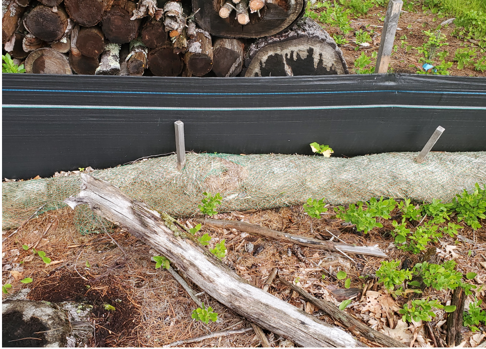
View of damaged silt wattle in northern portion of the Site — facing north
