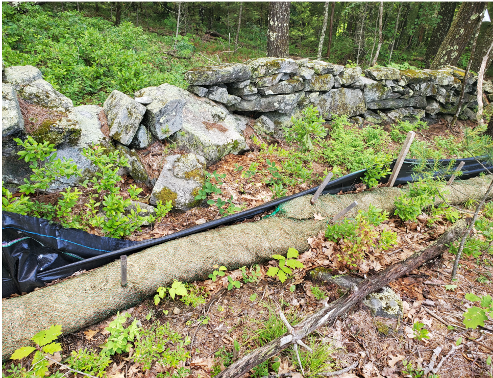
View of damaged silt fence in southeast portion of the Site — facing southeast
