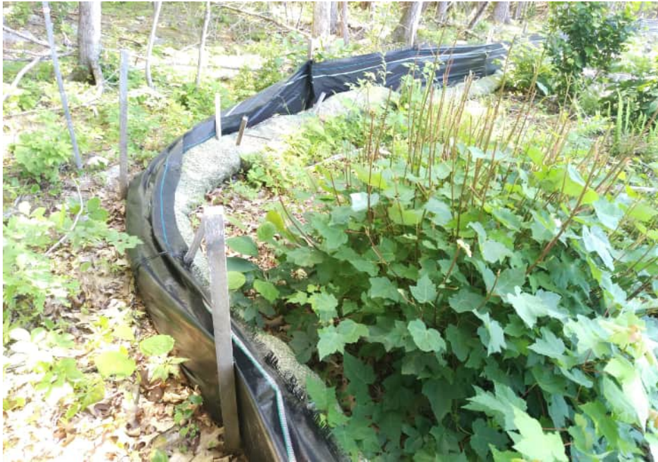
View of damaged silt fence in eastern portion of the Site — facing east
