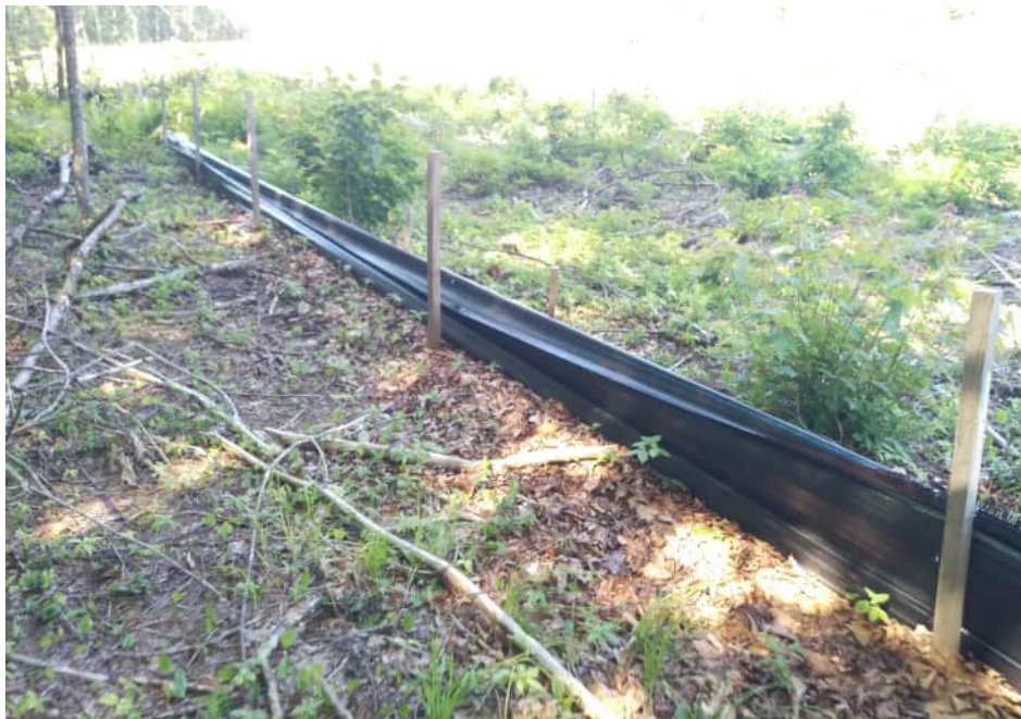
View of damaged silt fence in southeast portion of the Site — facing southwest
