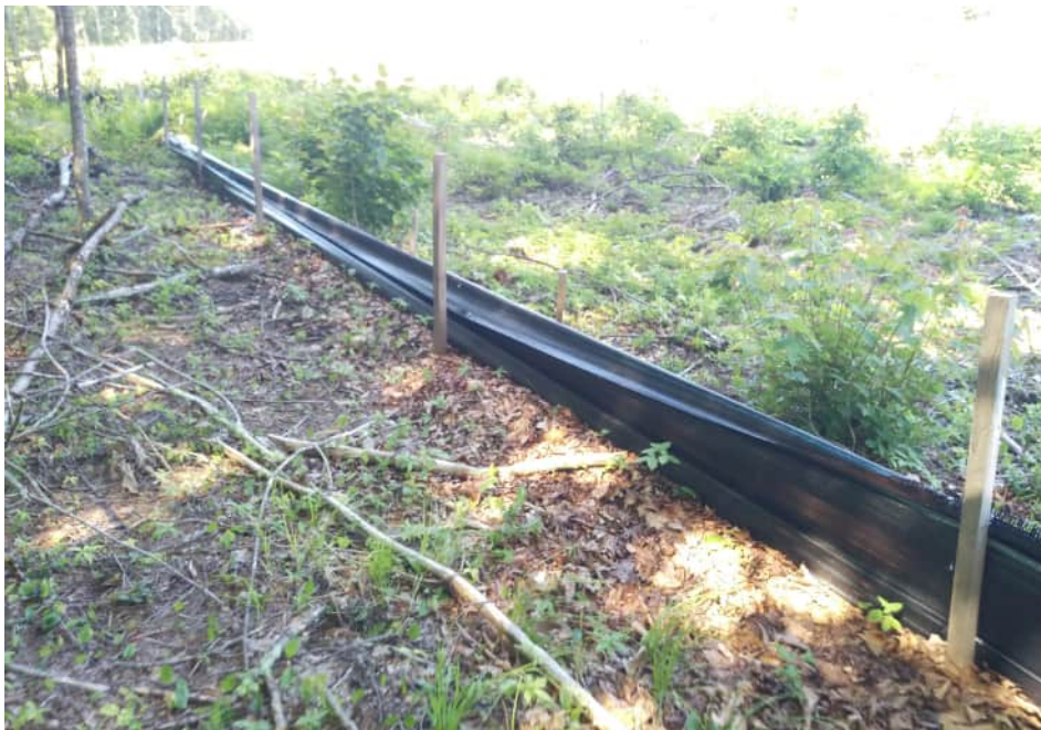
View of damaged silt fence in southeast portion of the Site — facing southwest
