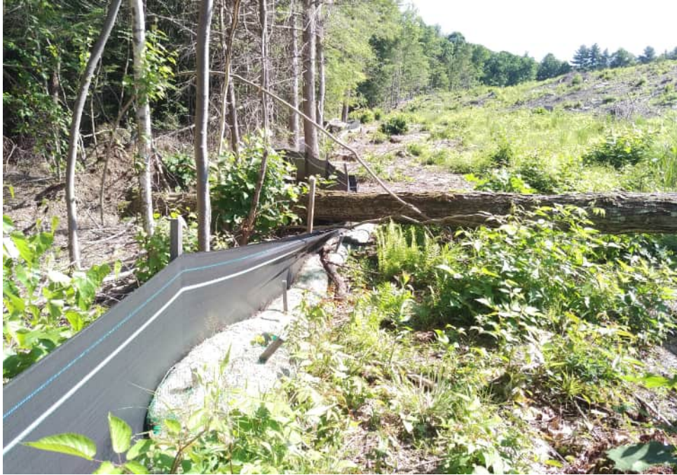
View of fallen tree damaged to silt fence in northern portion of the Site — facing east
