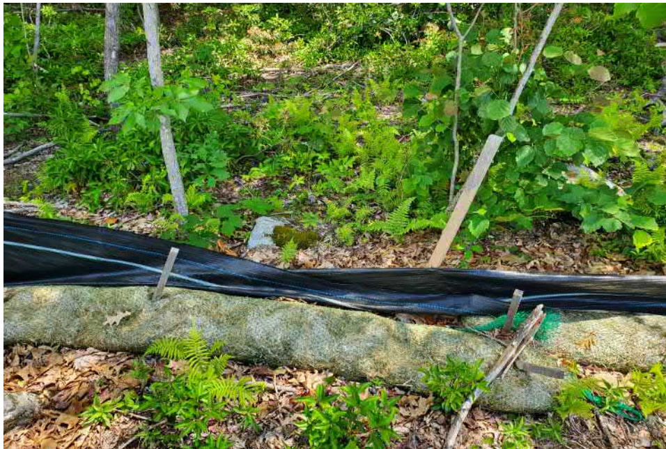
View of damaged silt fence in southeast portion of the Site — facing southeast
