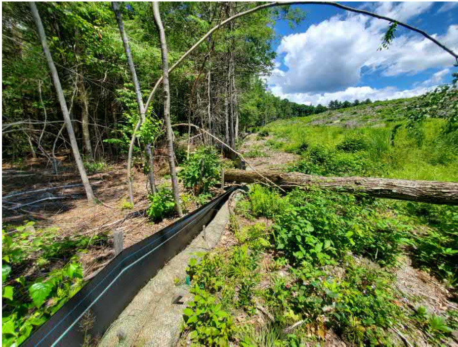
View of fallen tree damage to silt fence in southwestern portion of the Site — facing north
