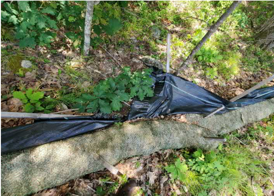
View of damaged silt fence in southeastern portion of the Site — facing southeast
