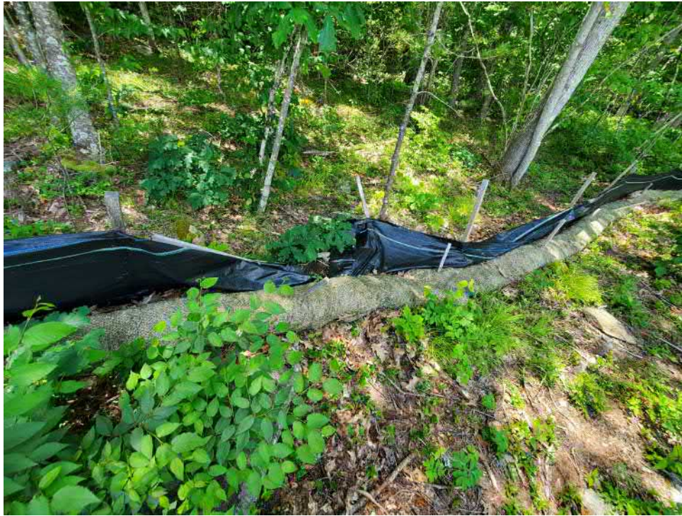
View of damaged silt fence in eastern portion of the Site — facing east
