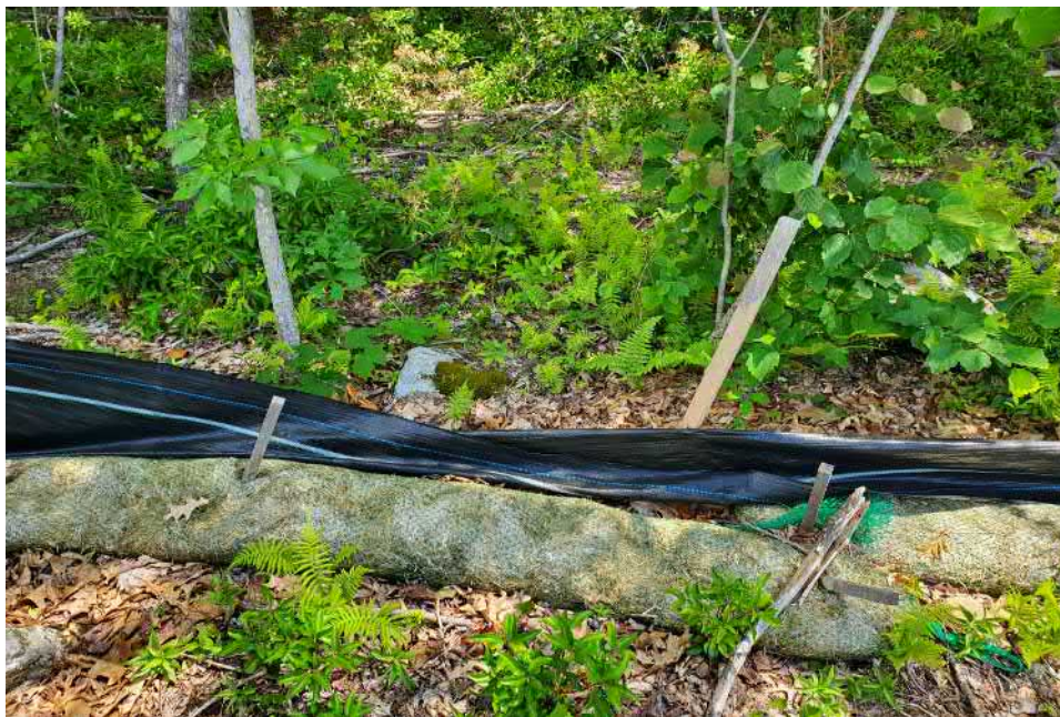
View of damaged silt fence in southeast portion of the Site — facing southeast
