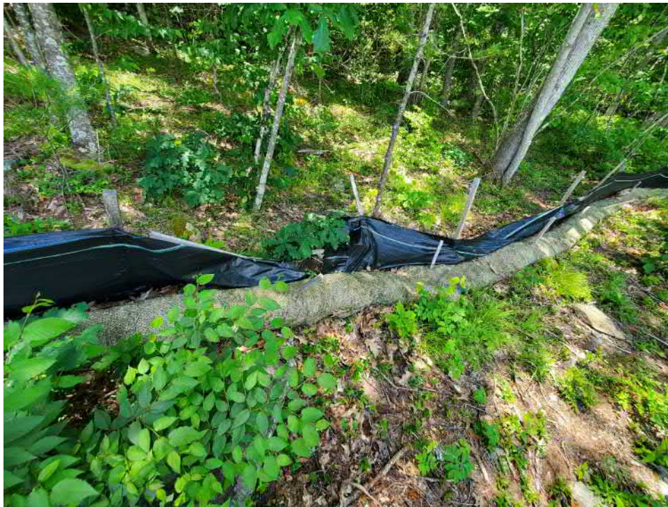
View of damaged silt fence in eastern portion of the Site — facing east
