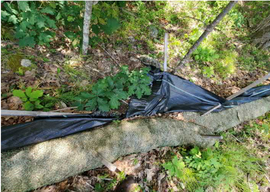
View of damaged silt fence in southeastern portion of the Site — facing southeast
