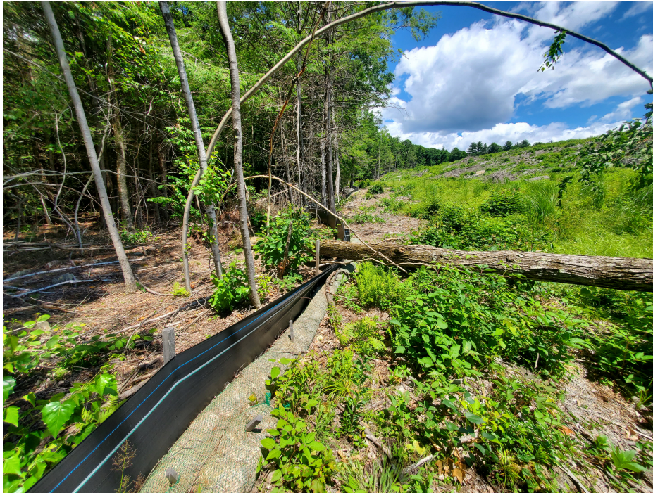
View of fallen tree damaged to silt fence in southwestern portion of the Site — facing north
