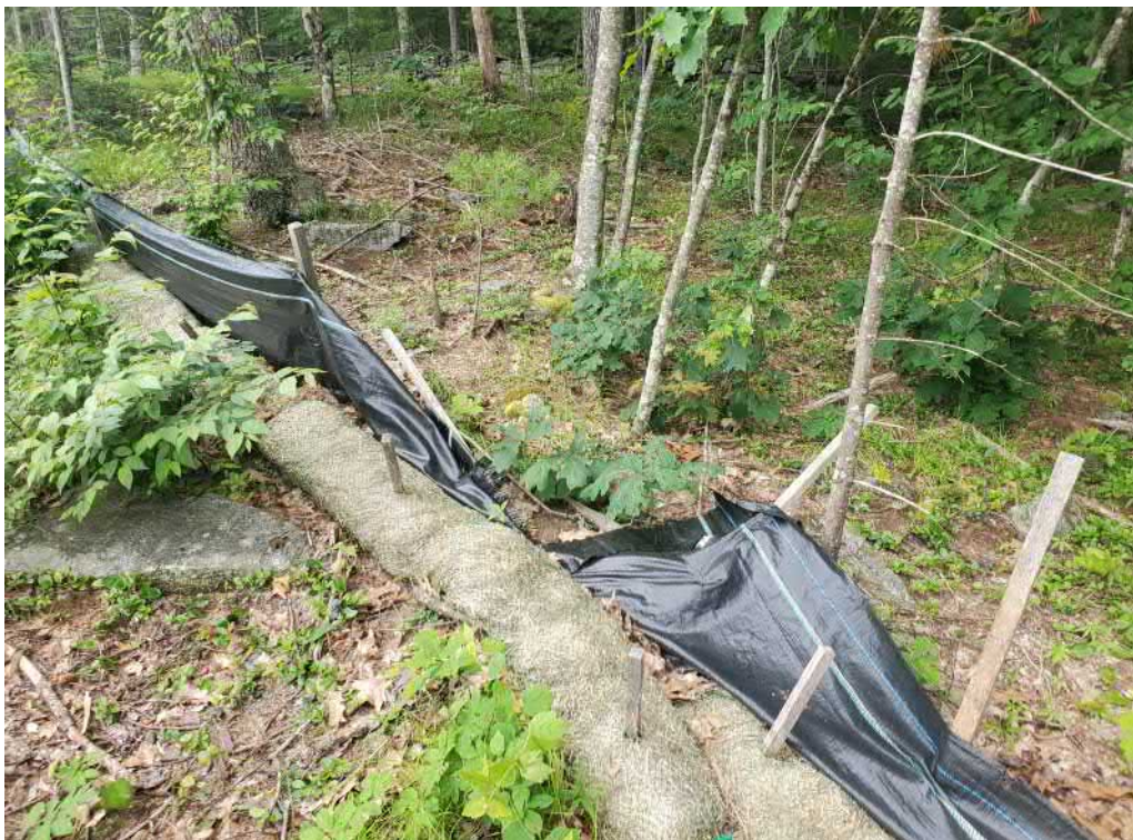
View of damaged silt fence in southeastern portion of the Site — facing northeast
