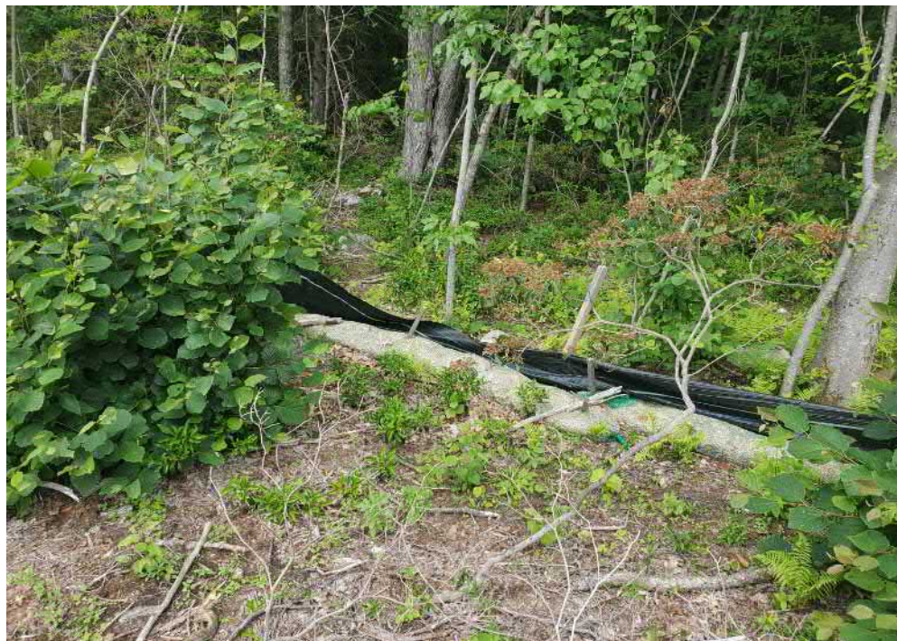
View of damaged silt fence in southeast portion of the Site — facing northeast
