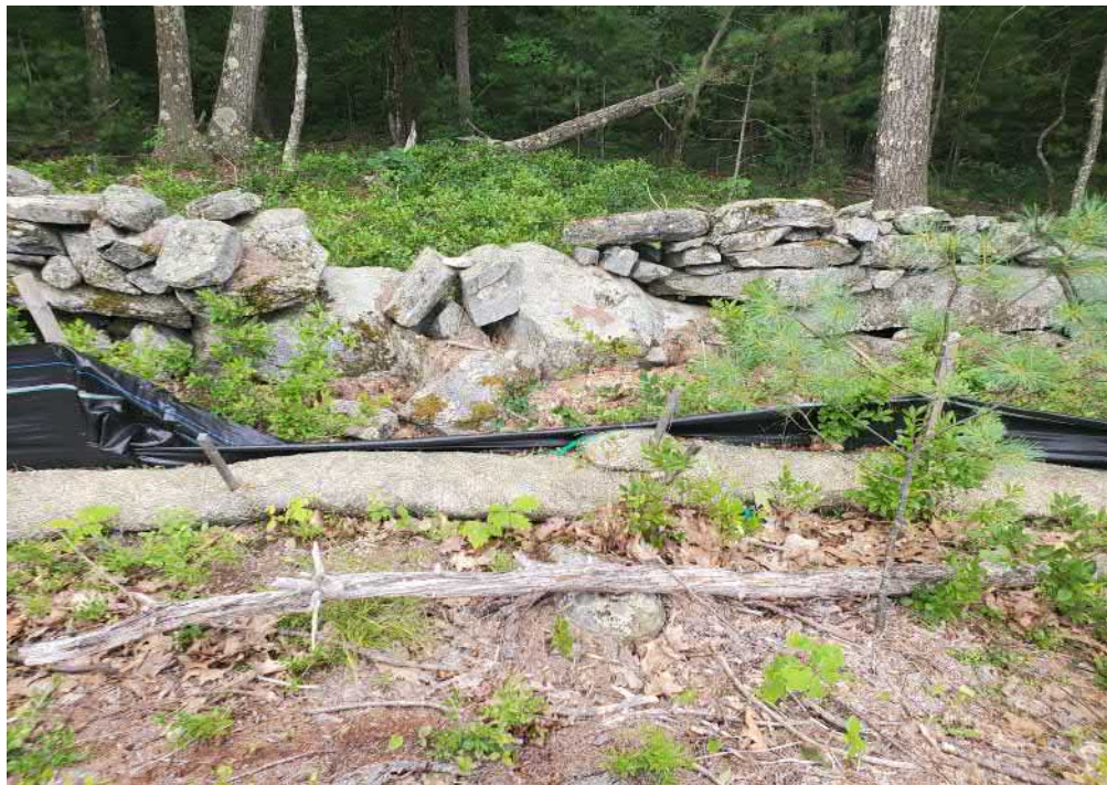
View of damaged silt fence in northeastern portion of the Site — facing east
