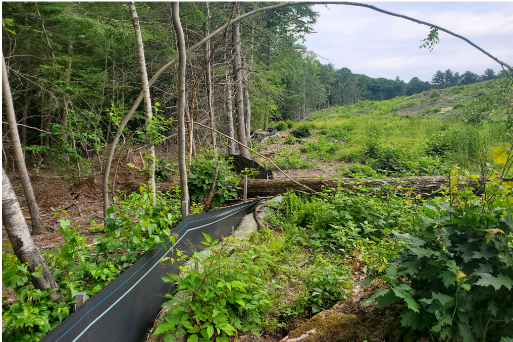
View of fallen tree damaged to silt fence in southwestern portion of the Site — facing north
