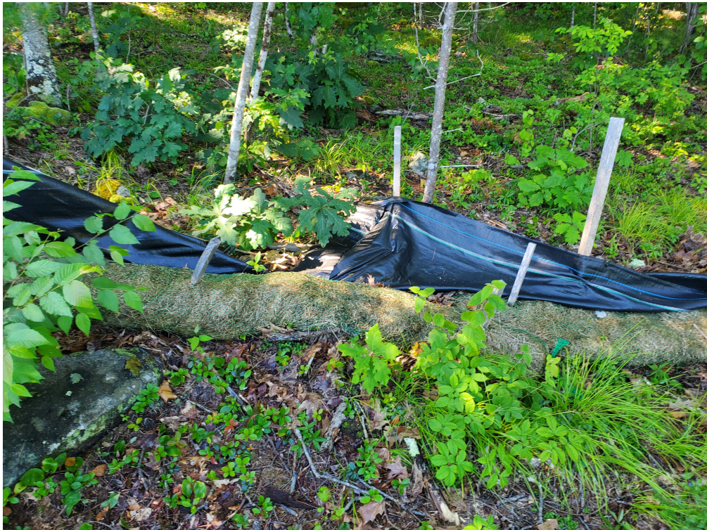
View of damaged silt fence in southeastern portion of the Site — facing northeast
