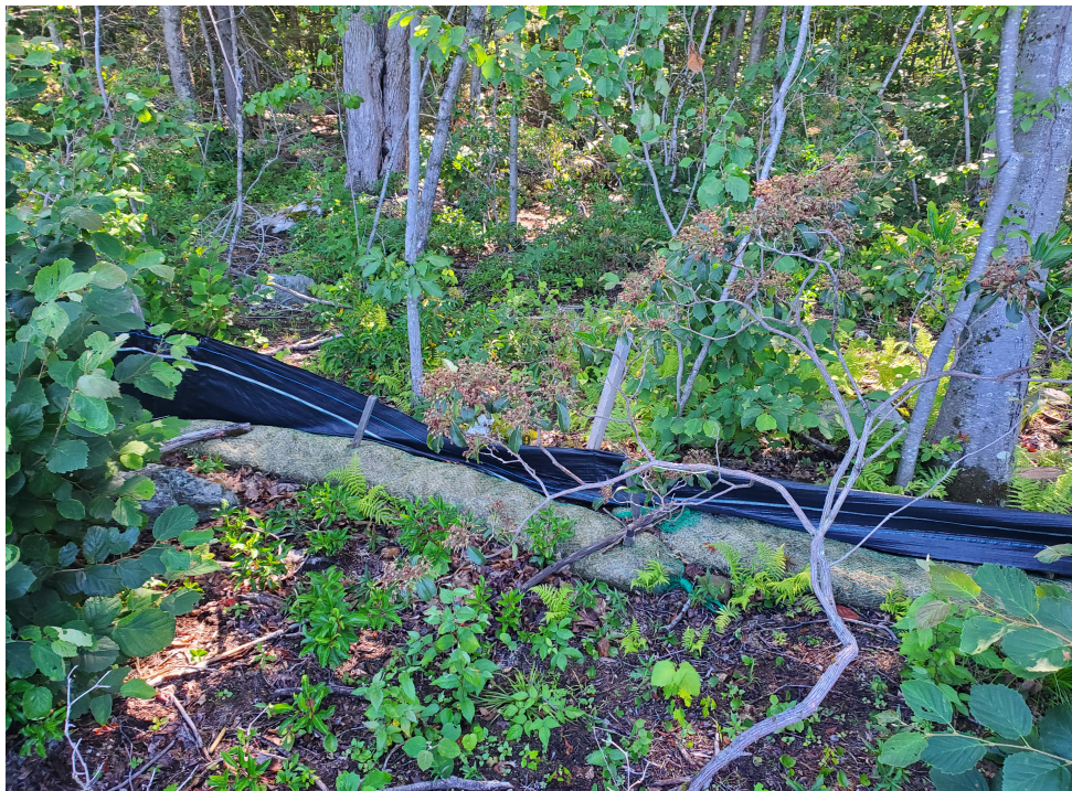
View of damaged silt fence in southeast portion of the Site — facing northeast
