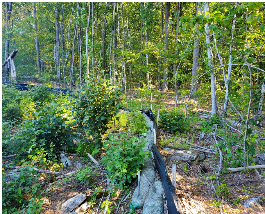
View of damaged silt fence in northeast portion of the Site — facing northeast
