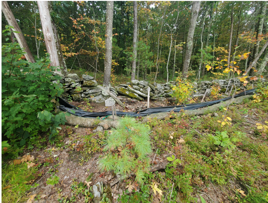
View of damaged silt fence in northeastern portion of the Site — facing east
