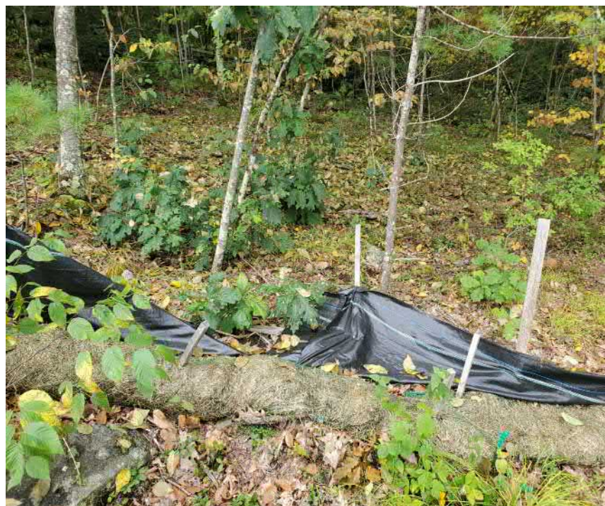
View of damaged silt fence in southeastern portion of the Site — facing northeast
