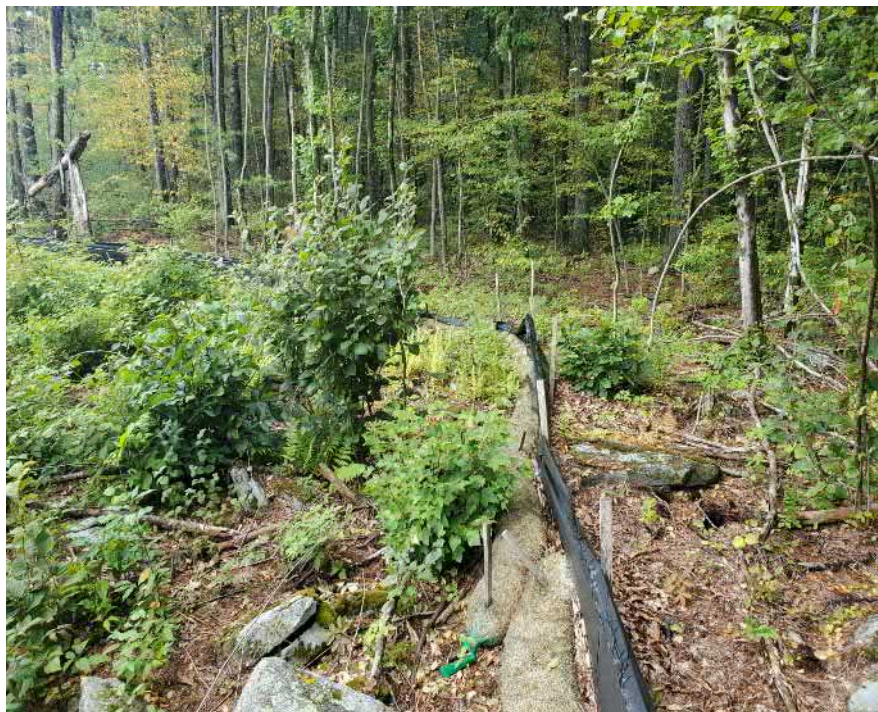
View of damaged silt fence in northeast portion of the Site — facing northeast
