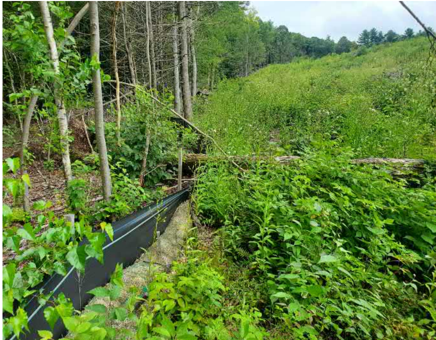
View of fallen tree damage to silt fence in southwestern portion of the Site — facing north
