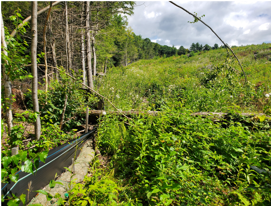
View of fallen tree damage to silt fence in southwestern portion of the Site — facing north
