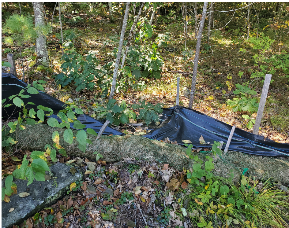
View of damaged silt fence in southeastern portion of the Site — facing northeast
