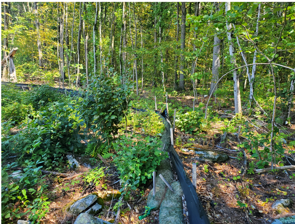
View of damaged silt fence in northeast portion of the Site — facing northeast
