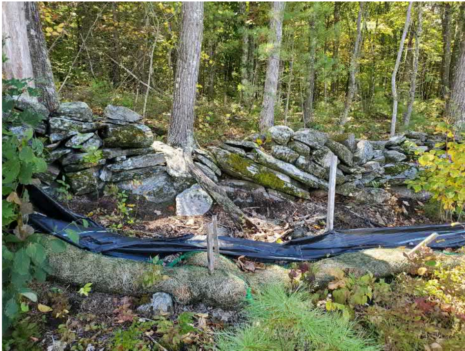
View of damaged silt fence in northeastern portion of the Site — facing east
