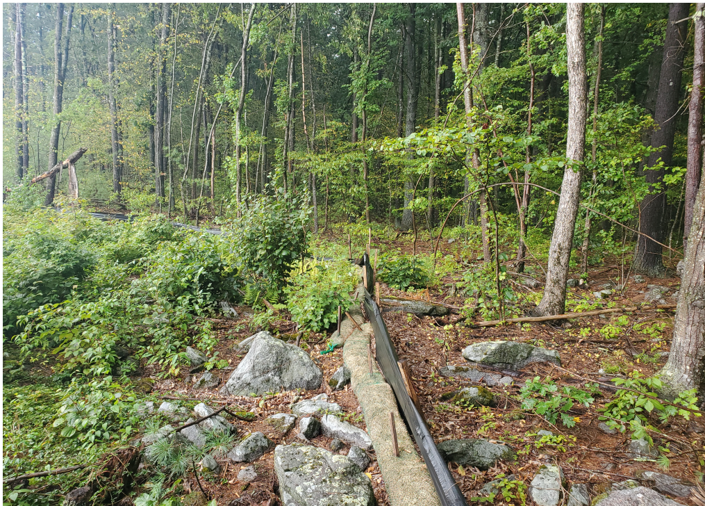
View of damaged silt fence in northeast portion of the Site — facing northeast
