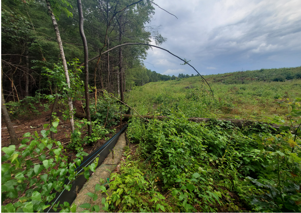
View of fallen tree damage to silt fence in southwestern portion of the Site — facing north
