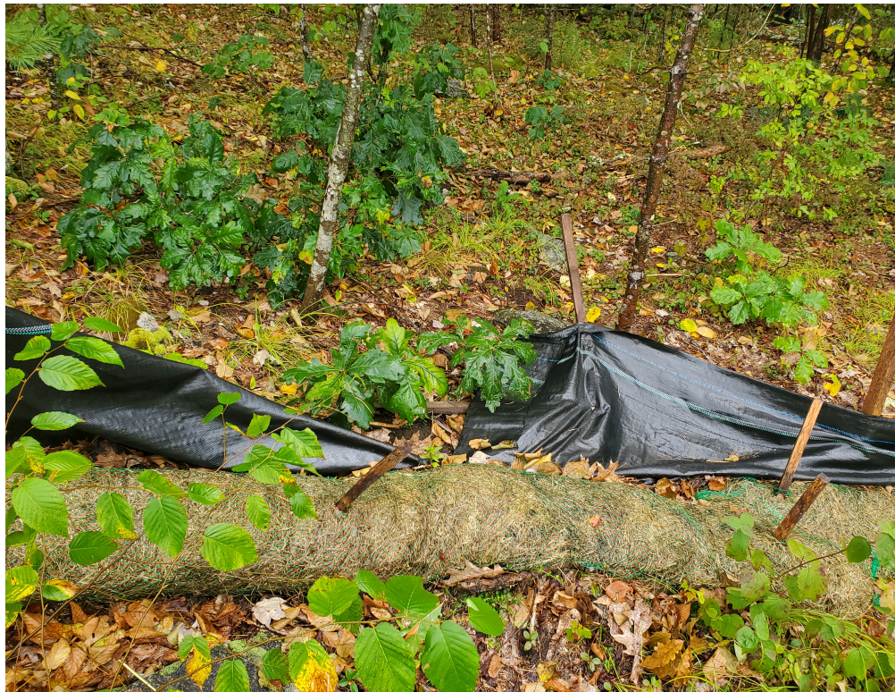
View of damaged silt fence in southeastern portion of the Site — facing northeast
