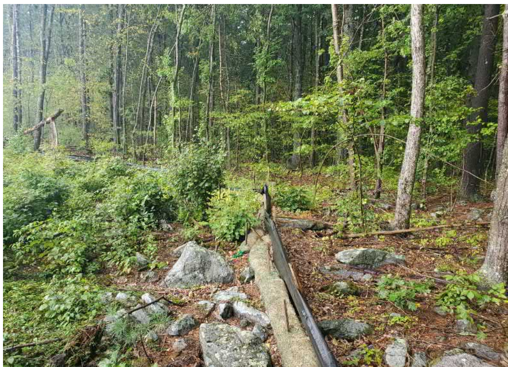
View of damaged silt fence in northeast portion of the Site — facing northeast
