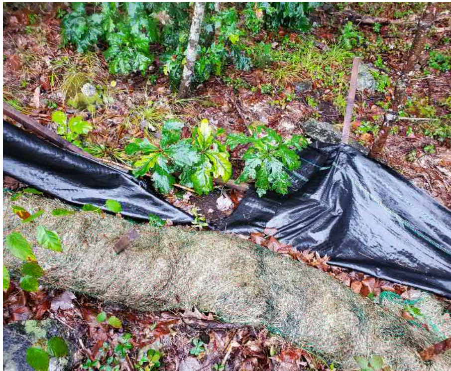
View of damaged silt fence in southeastern portion of the Site — facing northeast
