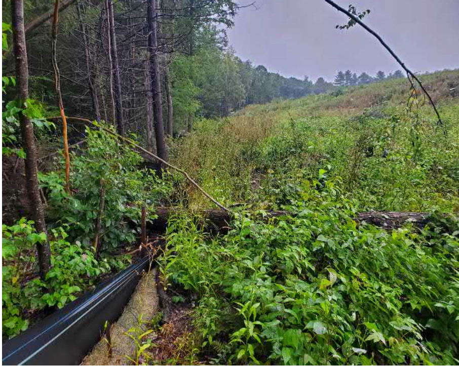
View of fallen tree damage to silt fence in southwestern portion of the Site — facing north
