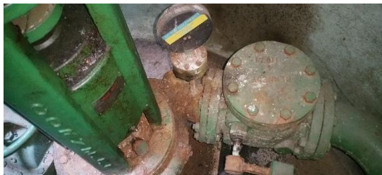
Photo: Leaking pump at Myles Standish PS
