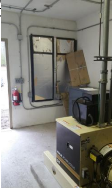
Photo: Blocked louver (Colt Circle PS)
