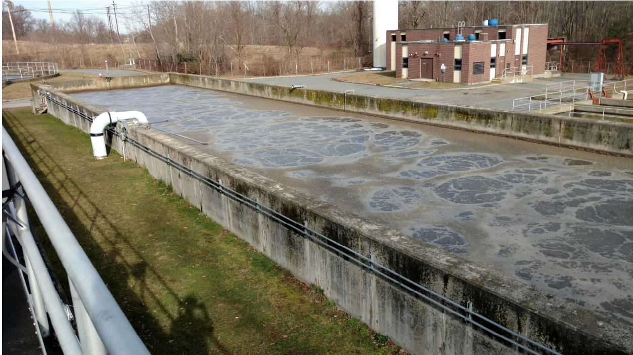
Figure 5-5 Diffused Aeration Tank
