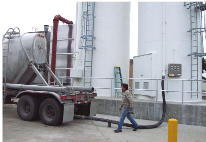
Typical Truck Unloading Station
