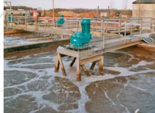
4 HYPERCLASSIC ® -Mixing & Aeration Systems in an industrial wwtP in Belgium (Food Industry)
