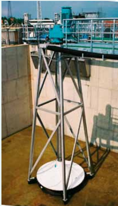
1 out of 9 HYPERCLASSIC®-Mixer/Aerators in an industrial wwtp in Belgium (Pulp & Paper Industry)
