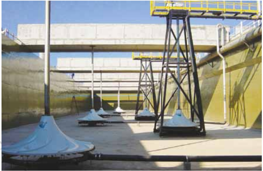
8 out of 22 HYPERCLASSIC® -Mixer/Aerators in a large municipal wwtp in São Paulo, Brazil
