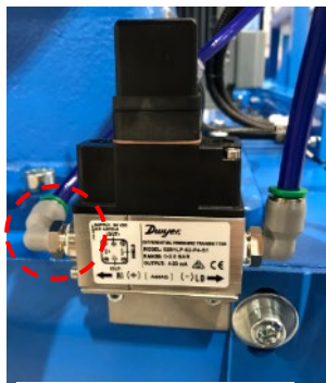
Figure 5 PDT-200 DP transmitter located near the gearbox. The blue tube/pipe is to be connected to the cone diffuser
