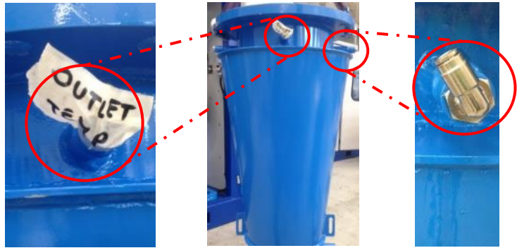
Discharge temperature transmitter & plastic tube/pipe
