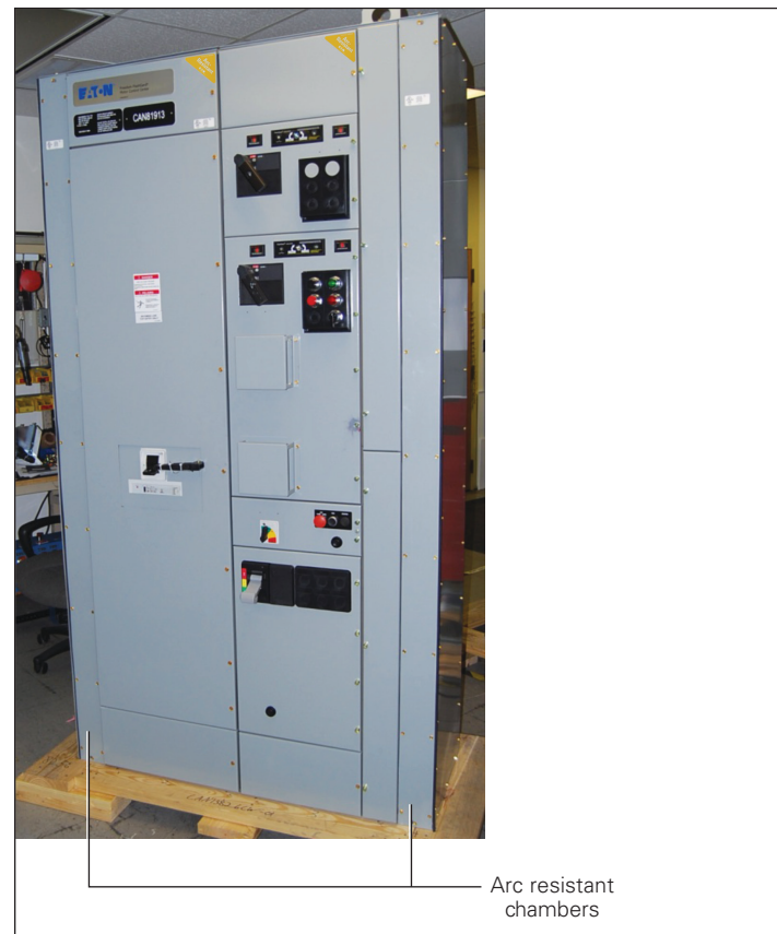
Figure 52. Arc resistant MCC lineup
