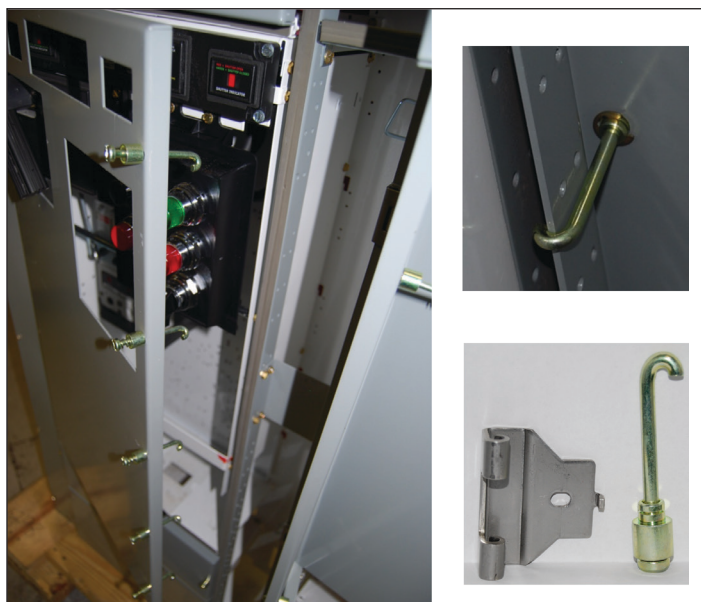
Figure 51. MCC unit and vertical wireway door latches and hinges
