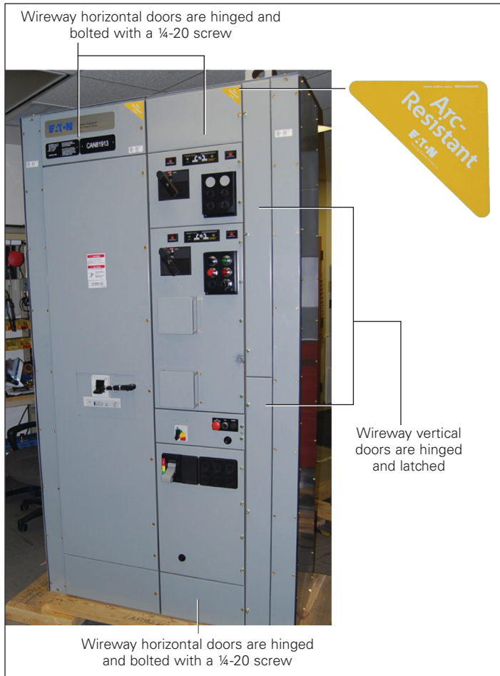
Figure 50. Arc resistant LV MCC—wireway doors and labeling
