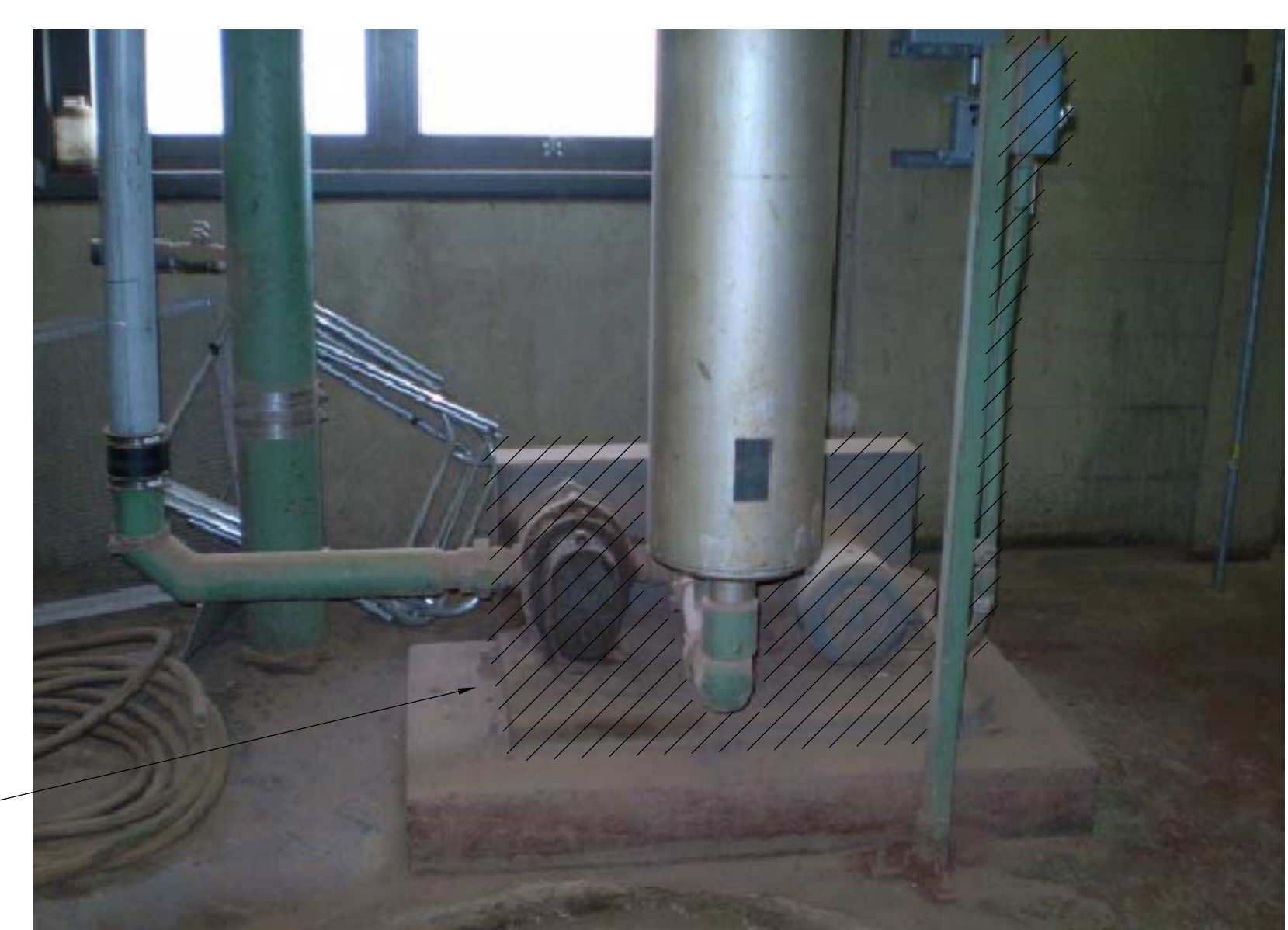
FLUIDIZING BLOWER PHOTO 1
